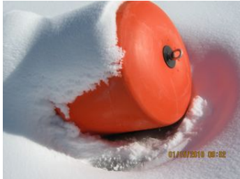
To right is float attached to intake of 12-inch outfall hose with a four-foot length of chain. The float appears to be resting on reservoir bottom at edge of withdrawal sump.
